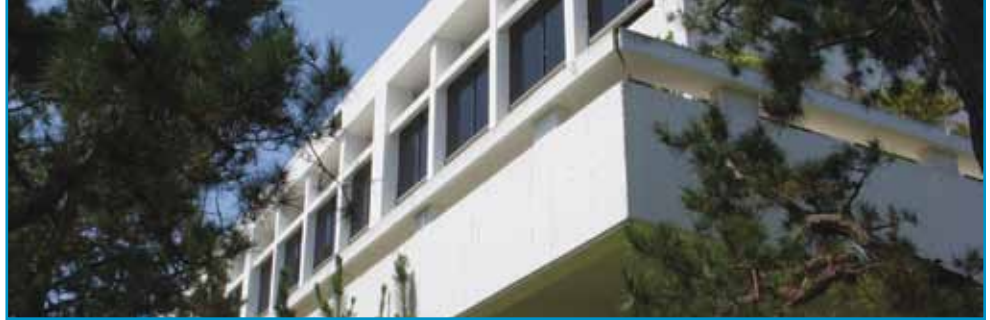
Building M5, southeast corner showing dramatic cantilevered post-tensioned beams at Plaza Level. Courtesy of Phillip Yee of Northrop-Grumman.
